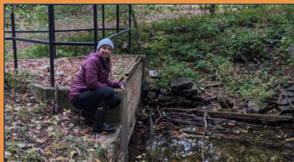
Little Lake outlet structure
